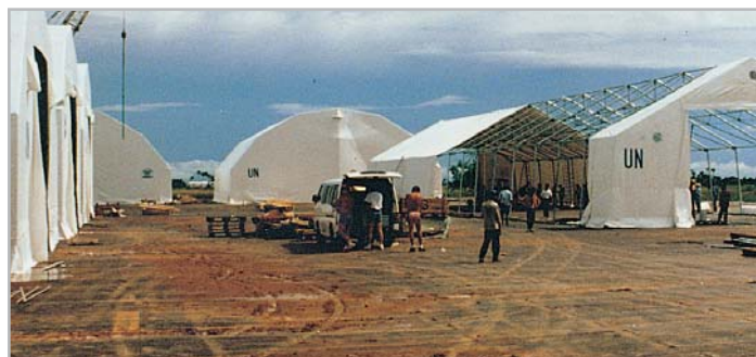
A total of 98 hangars, workshops and stores were supplied to the United Nations for this relief camp in Cambodia
