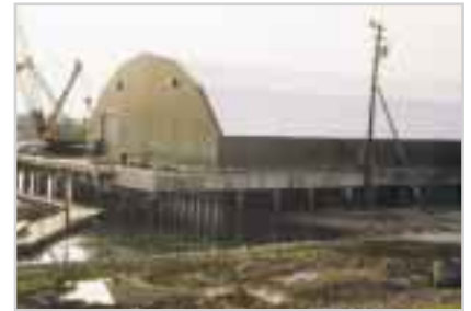
Above: Merrill Marine Terminal, Portland, Maine USA. This recycled paper storage building was back in business with a new membrane roof one week after a major fire in 1999. The self-venting properties of the roof membrane enabled the building frame to survive an extreme fire with no structural damage.
