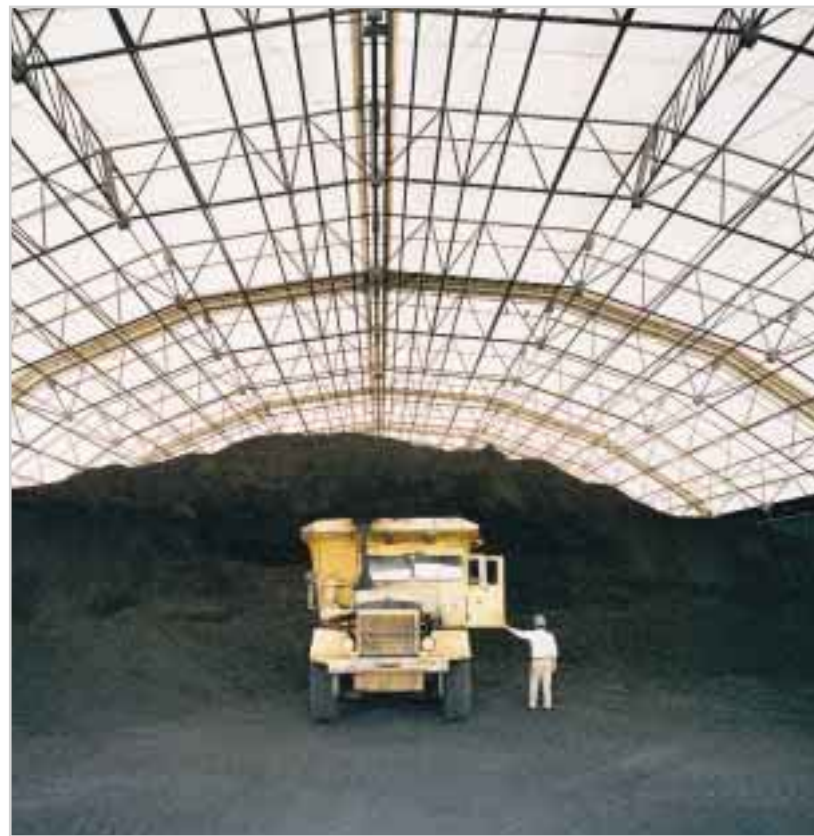
Below: Merrill Terminal, Portland, Maine, USA. Translucent roof membrane provides excellent working conditions during day light hours. Rubb structures accommodate large bulk material handling equipment for efficient movement of materials.
